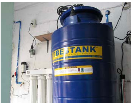
The filtration system
