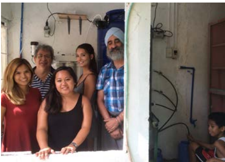
The UH Group at the Site After Installation (the child on the right is filling his water cans from the faucet)
